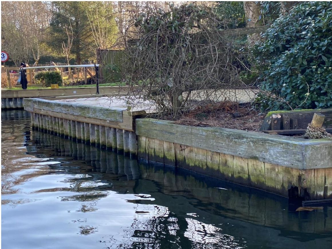
Above: Steel (left hand side) and timber (right hand side) quay heading, both with timber whaling boards and capping.
