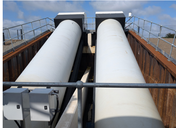
A new drainage pump at Norton's on the Yare helps manage both flood protection and water retention, supporting the carbon-rich floodplain and nature conservation. Andrea Kelly
